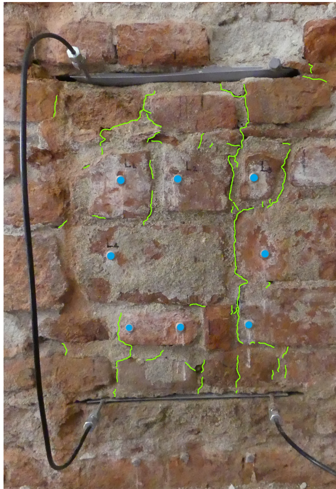
Figure 2.7: The picture shows a double flat jack test. This photo was taken at the end of the test. In the picture, the measure points are highlighted in blue and the cracks in green. Position 1 "ex Teatro dei Nobili".
