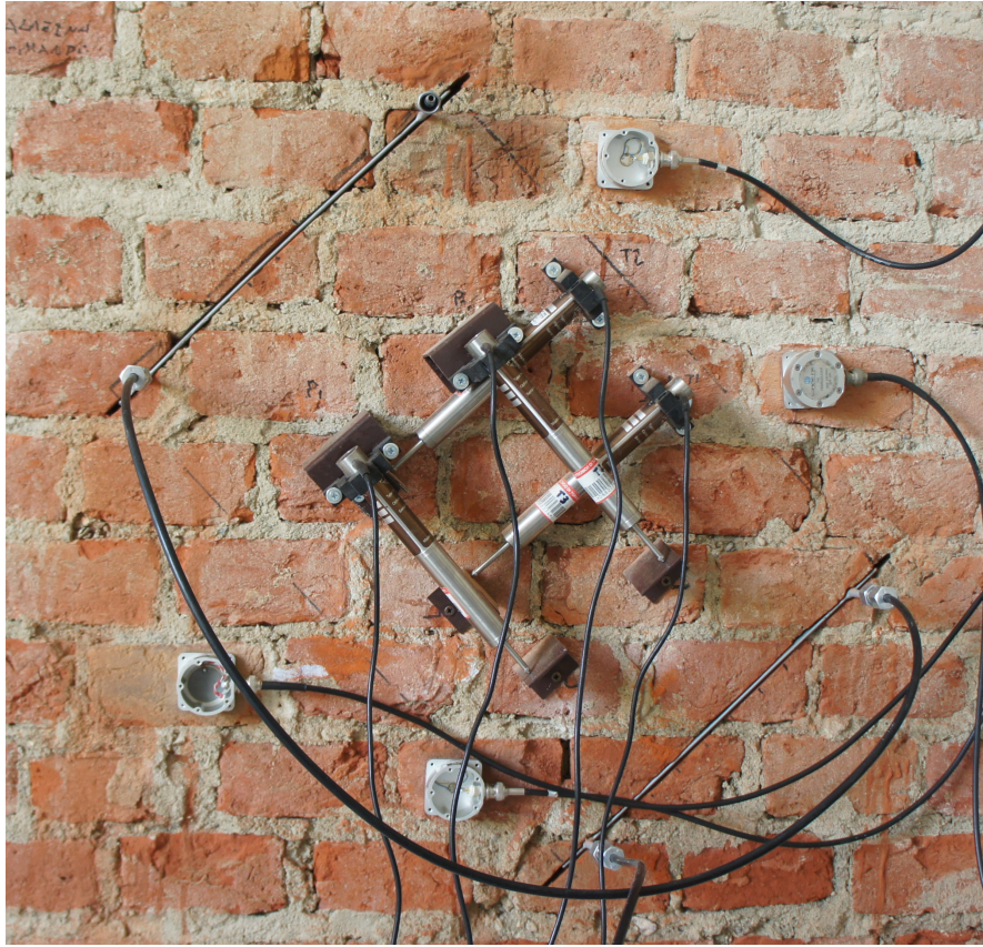
Figure 4.26: The image displays the set-up of the shear FJ test performed in the Command building.
