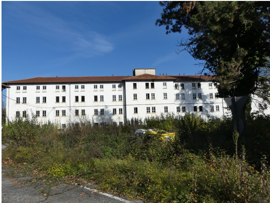
Figure 4.11: In the image a picture of the "Caserma Giovanni Cerutti" is shown.
