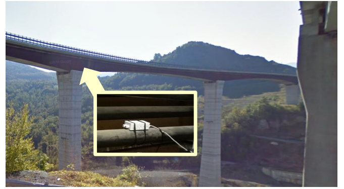
Fig. 8. Viaduct along an Italian motorway, where sensors deployed for structural health monitoring are attached to the internal tendons.
