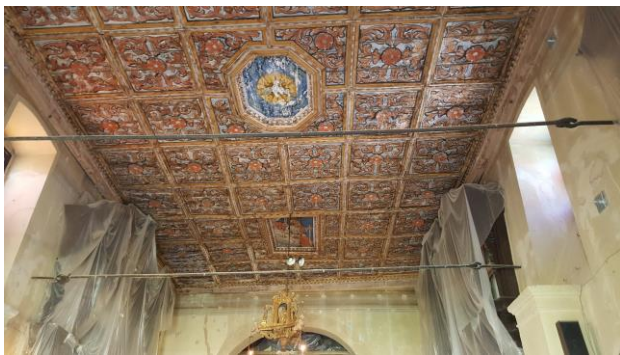
Figure 1. The coffered painted wooden ceiling of the sanctuary of S. Maria delle Grazie church in Varoni (Amatrice - RI), after the 2016 earthquake.
