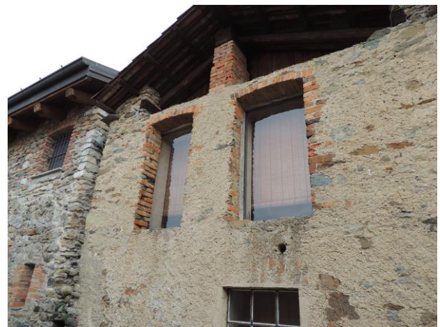
Figure 16. Building F - Intervention preserving both the external masonry surfaces and the roof (credits Silvia Rescic).
