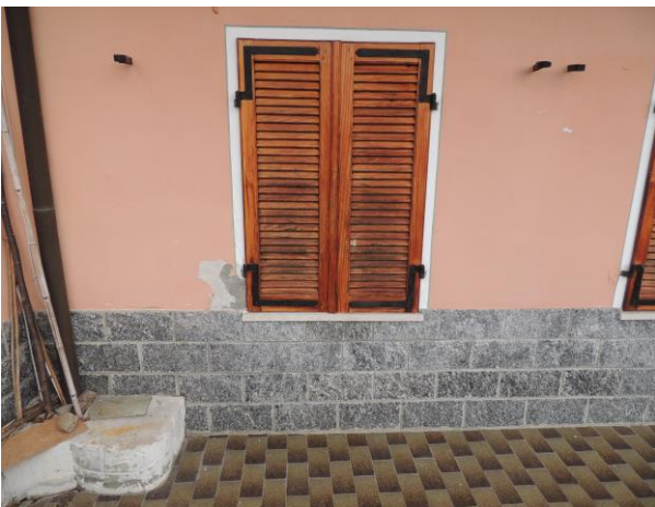
Figure 8. Building E - Baseboard in stone slabs and an external flooring in ceramic tiles, replacement of the windows and application of a new finishing layer (credits Fabio Fratini).
