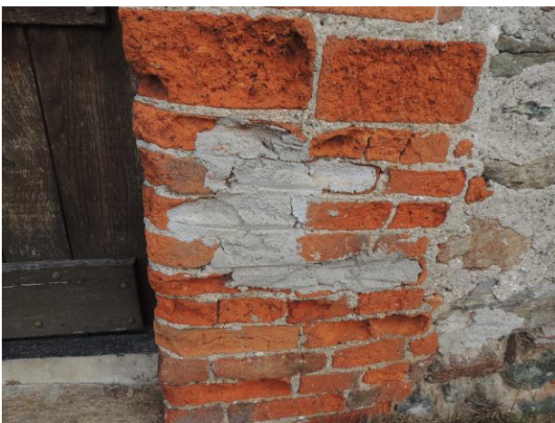
Figure 14. Building A - Reintegration of eroded bricks with cement mortar (credits Fabio Fratini).
