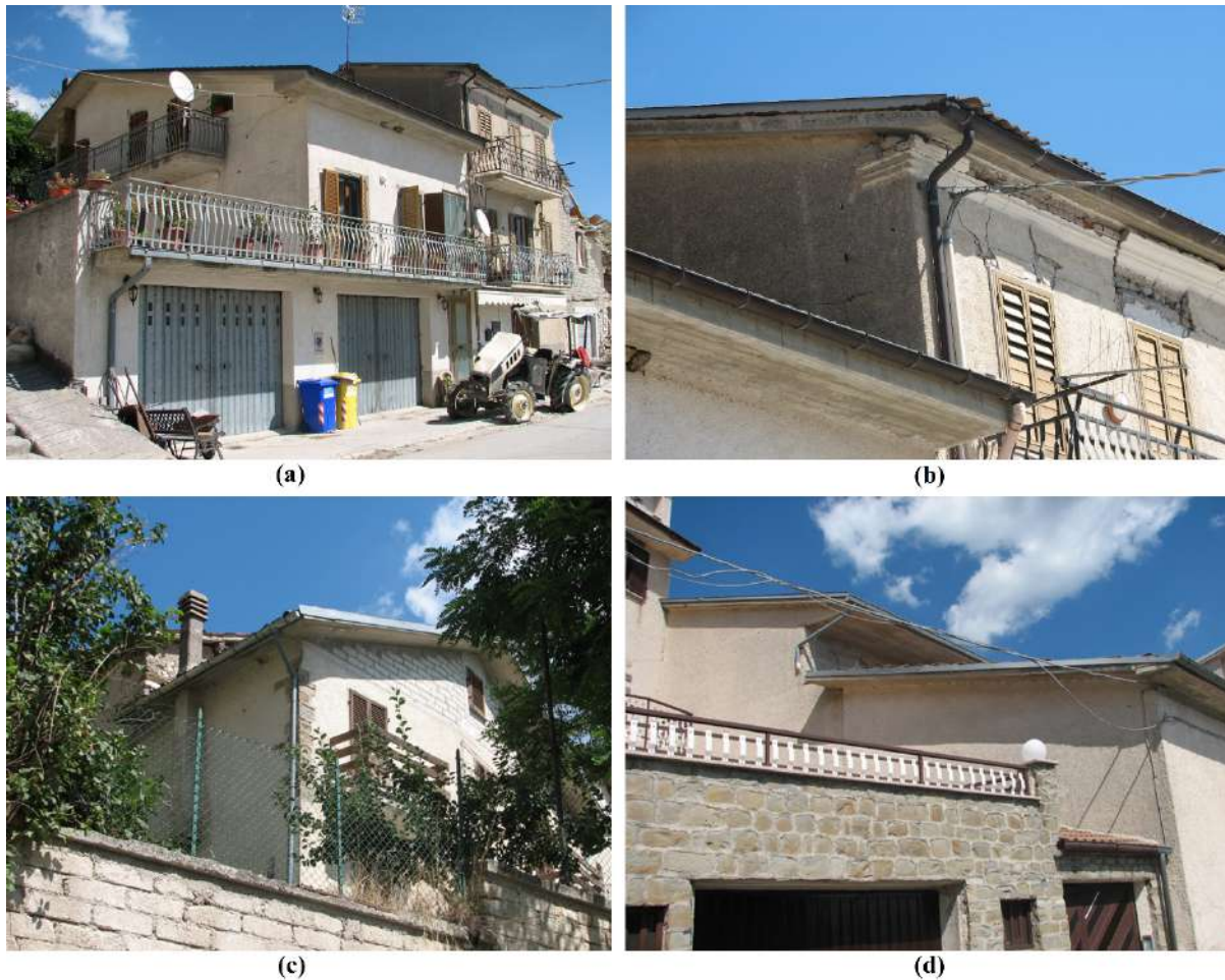
46 47 Figure 1. Masonry buildings retrofitted with concrete roof not collapsed after the earthquake in 48 Pescara del Tronto (a-b) and small villages near Accumoli (c-d).
