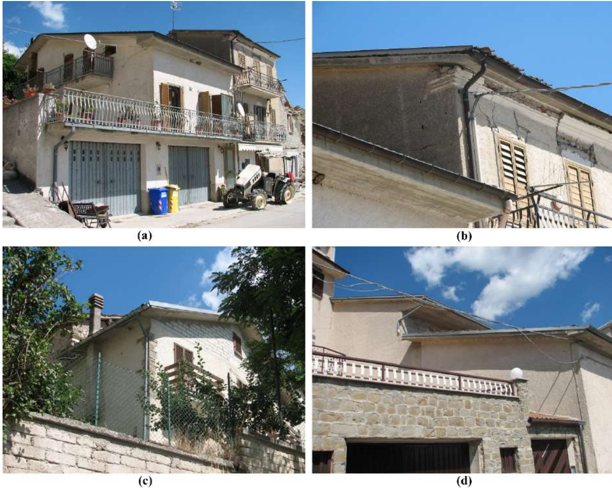
46 47 Figure 1. Masonry buildings retrofitted with concrete roof not collapsed after the earthquake in 48 Pescara del Tronto (a-b) and small villages near Accumoli (c-d).
