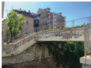
Via Saint Bon: The old passage of the train that went to Porta Palazzo has been abandoned and the area is in a very poor condition. Both the public space and the housing buildings are deteriorated; the lack of surveillance has made the area a dump.
