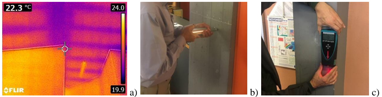
Figure 5: a) Constructional element identification using thermal camera; b) data acquisition with sclerometer; c) Measurements with pacometer
