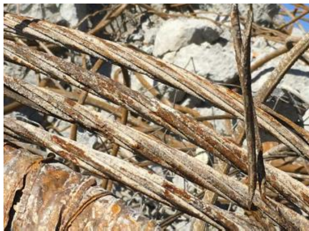
Figure 2. Pitting corrosion of prestressing tendons.
