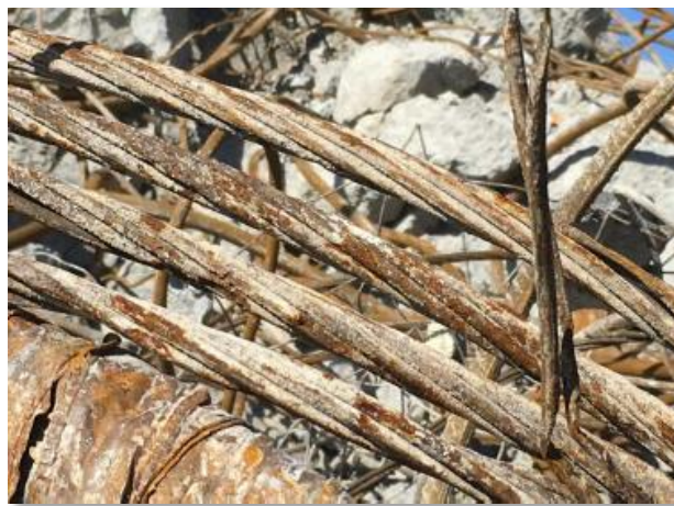
Figure 2. Pitting corrosion of prestressing tendons.
