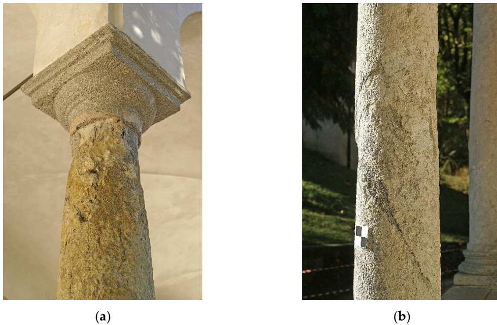
Figure 7. Different types of surface material degradation on the columns of the Via Crucis portico: (a) erosion; (b) exfoliation.
