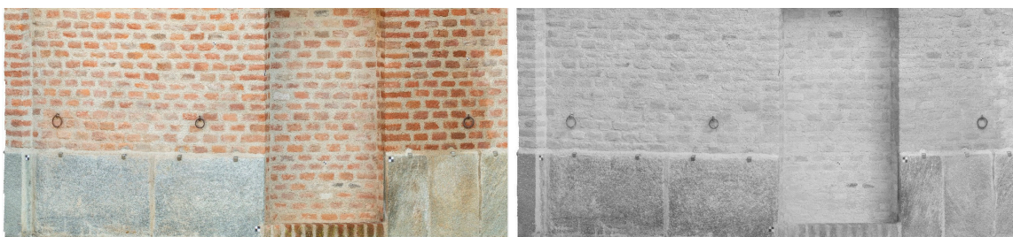
Figure 12. Comparison of details from the VIS (left) and NIR (right) dataset 2 textured models to evaluate identification of bio-deterioration on the façade's surface.
