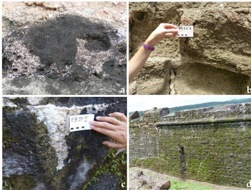
Figure 4. Pictures representing several deterioration processes observed at the sites. (a,b) at Panamá Viejo, (a) biological growth; (b) surface recession/material loss; (c) encrustation at Fort San Fernando (Portobelo); (d) biological growth at Fort San Lorenzo.
