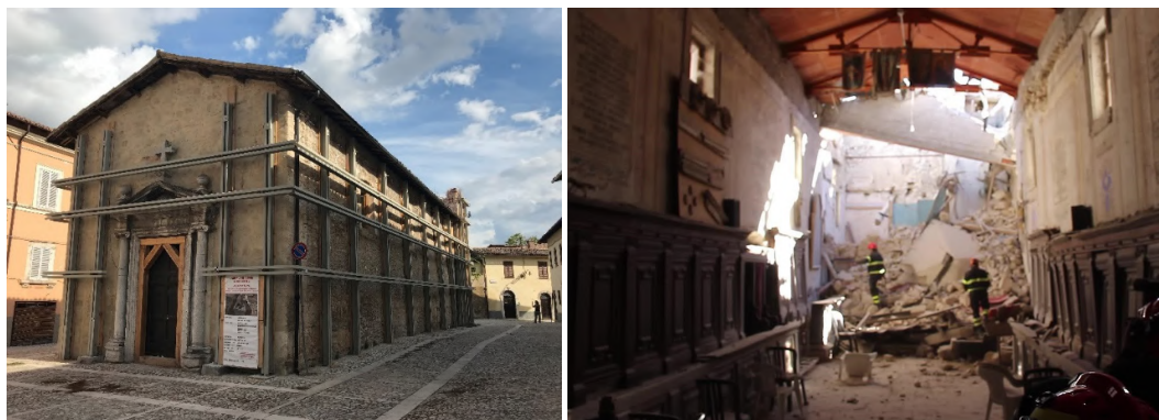
Figure 2. The Church of San Lorenzo in Norcia after the damage of the earthquake.
