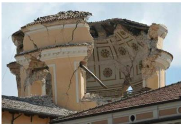
Fig. (2). Dome and drum of the Anime Sante Church in L'Aquila after the earthquake of 2009.
