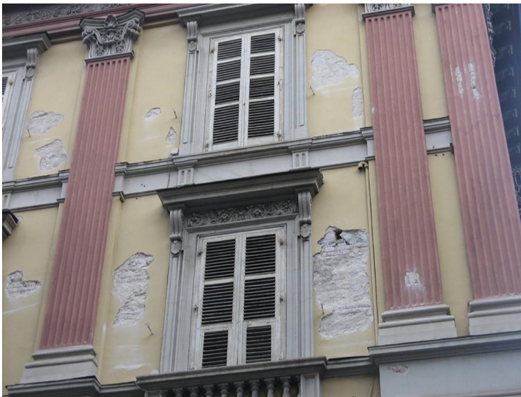
47 Fig. 2. Example of the mechanical incompatibility of patches made by cement mortar in a historical plaster 48 based on lime mortar. The noticeable difference in stiffness of the concrete patch against the original lime- 49 based plaster has favored the detachment under thermo-hygrometric stress. 50
