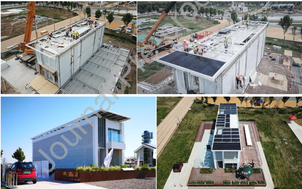
Figure 1: The LONG PLAN house during construction (top) and at the end of construction (bottom)
