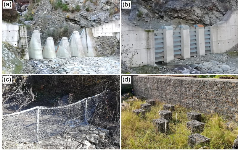
Figure 1: Examples of debris flow mitigation structures, with energy-breaking or filtering function. (a) Front breakers and (b) slit-filter barrier installed in Pollein, Aosta Valley, Italy. (c) Flexible steel-ring net installed in Bussoleno, Piedmont, Italy. (d) Debris-resisting baffles near Yu-Thung Road, Hong Kong, HKSAR.
