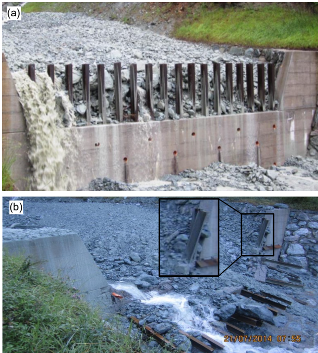
Figure 2: The filter barrier installed in the Grand Valey experimental site. (a) Picture of the intact barrier and (b) immediately after the collapse in 2014. Pictures courtesy of the Aosta Valley Regional Government.
