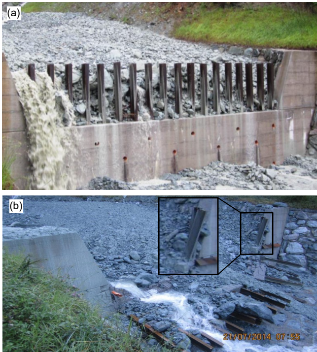
Figure 2: The filter barrier installed in the Grand Valey experimental site. (a) Picture of the intact barrier and (b) immediately after the collapse in 2014. Pictures courtesy of the Aosta Valley Regional Government.
