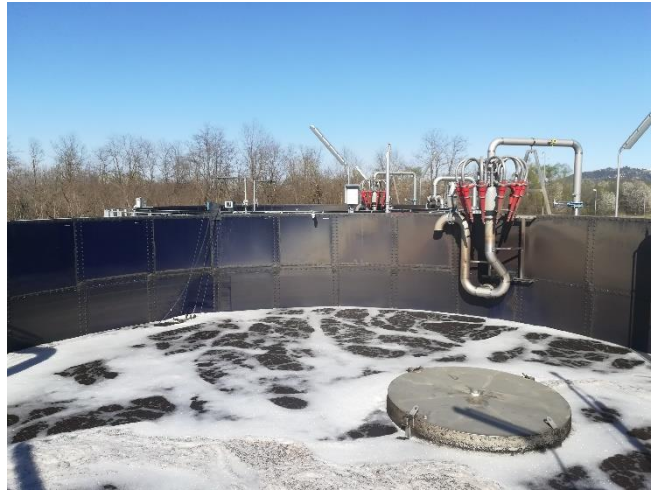
Figure 1. 8 Deammobification Unit. Demon. Castiglione Torinese WWTP- Smat
