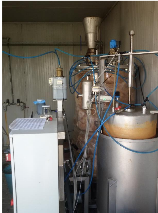
Figure 5. 2 Employed pilot anaerobic digester
