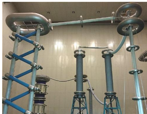
Fig. 14. \pm 500\text{kV} DC terminations under type test
