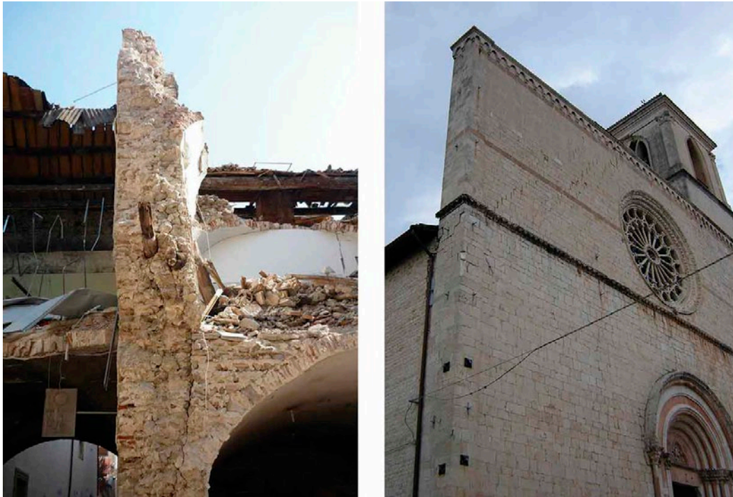
Fig. 1. L'Aquila: wooden log ( radiciamento ) in a shear wall (on the left). L'Aquila: the effectiveness of wooden logs inserted in the façade of the church of S. Silvestro preventing its global overturning (on the right).
