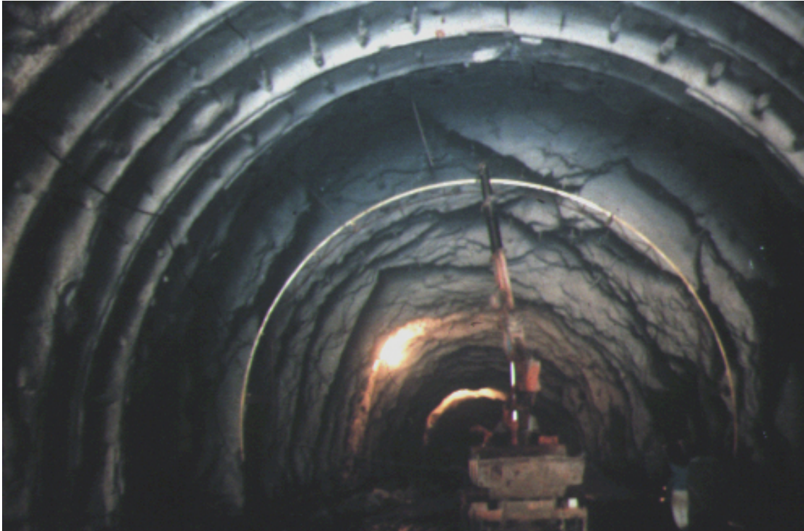
Fig. 3. Photograph of large overbreaks induced by joints discontinuities around a road tunnel. The steel rib indicates the theoretical tunnel boundary (courtesy Prof. S. Pelizza).
