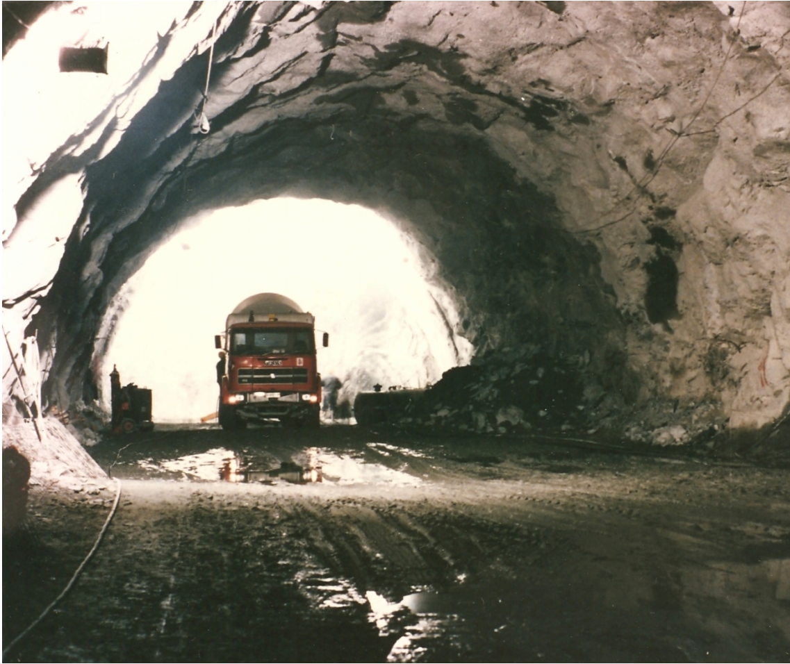
Fig. 4. Example of usual irregularity of the boundary for a road tunnel excavated by drill and blast in black calcareous shists (courtesy Prof. S. Pelizza).
