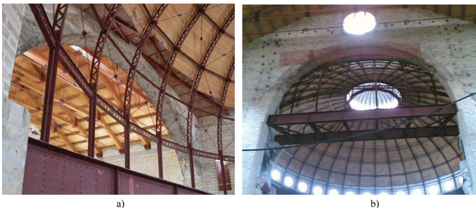
Figure 8. Photographs of the view of the dome bracing system (a), and the dome support to the girder and to masonry (b).
