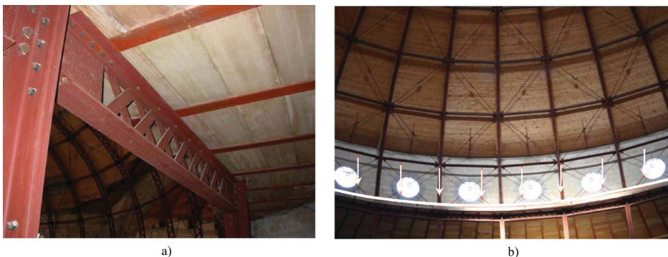
Figure 11. Photographs of the present configuration of the floor around the base of the steel dome (a), and localization of the string course at the concrete floor level (b).
